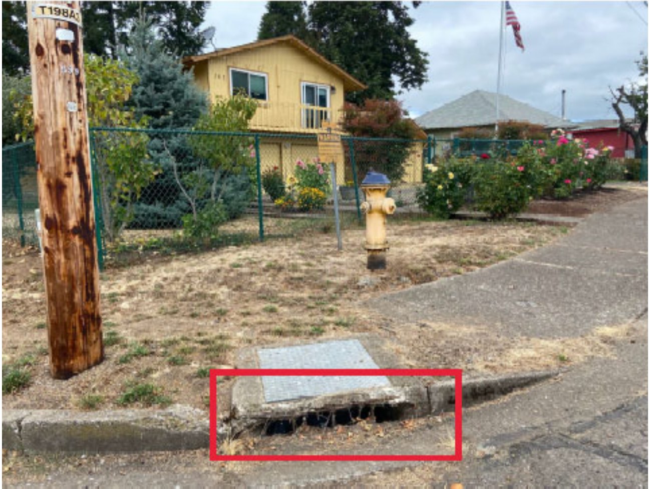
Figure 6: Curb Inlet Cross Connected to Sewer System; Corner of Moss and Lakeview
